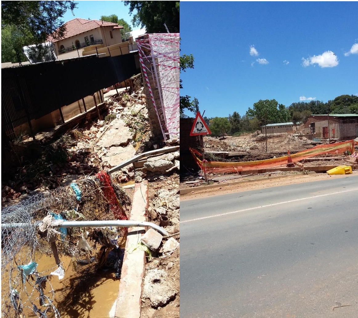
The culvert going north (down stream) from Louis Rd, Looking south from Louis Rd into the Paterson Park site.
