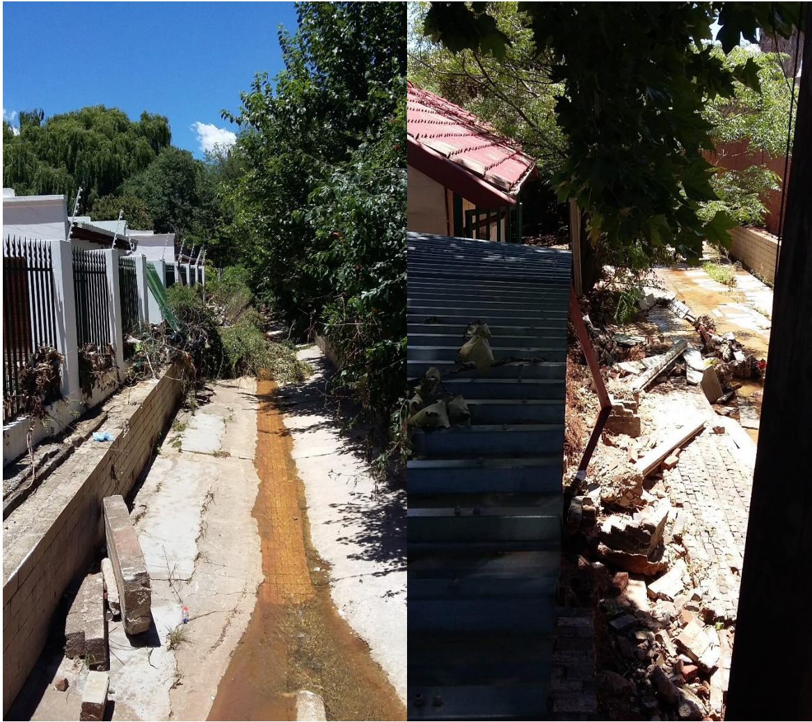
General views of the culvert showing large bits of wall that had been dumped from further up as well as a boundry wall that was pushed over into the culvert by water coming in laterally.
